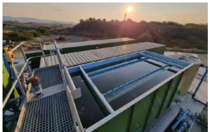
Newly constructed reverse osmosis plant
