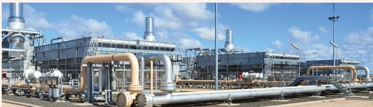
Wallumbilla Compressor Station in Queensland
